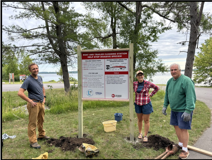
George Seifried (ESLA Vice President), Michael and Samantha Ogle install sign at the Baggs Road Launch on Skegemog.
